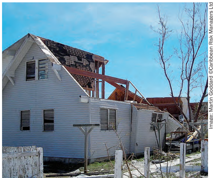
Damage on Grand Turk, in the Turks & Caicos Islands, after the passing of Hurricane Ike in 2008
