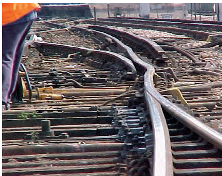
Increasing summer temperatures take their toll on existing rail infrastructure
