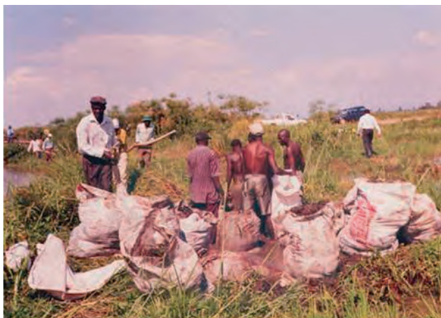
Nyando community using sand bags to block eroded Nyando river bank
